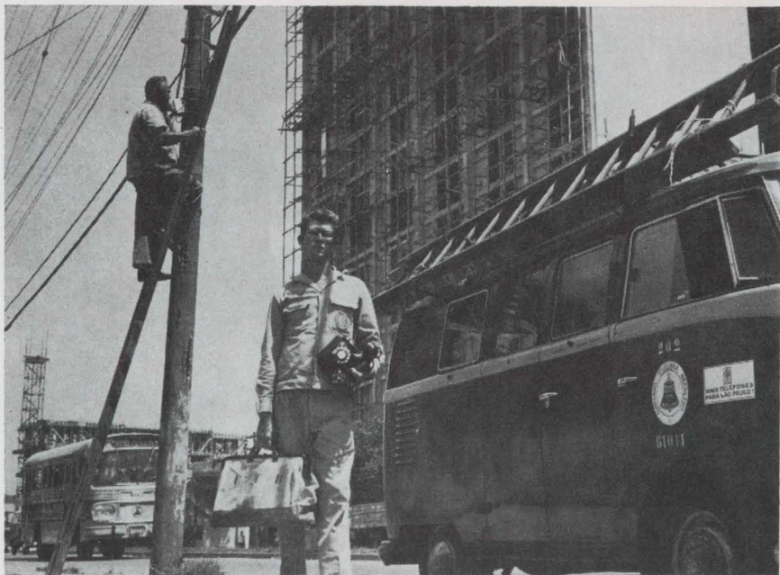
Utility. A key element in Brazil's drive to improve internal communications is the installation of 1.1 million new telephone lines in its major cities.
