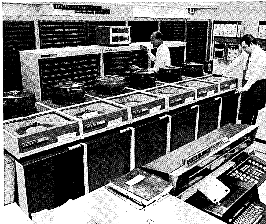
The on-line CDC 3300 processor stands back to back with another as one of the precautionary measures taken by Hornblower.
