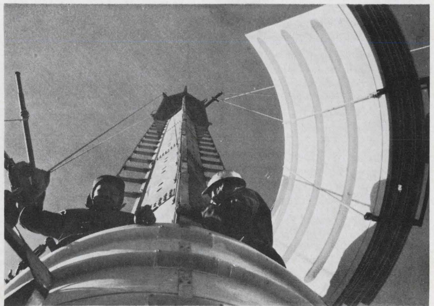
View from the top. Stack of 18 arrays with four radiators each makes up tv antenna inside cylindrical shield at top of Munich tower.
